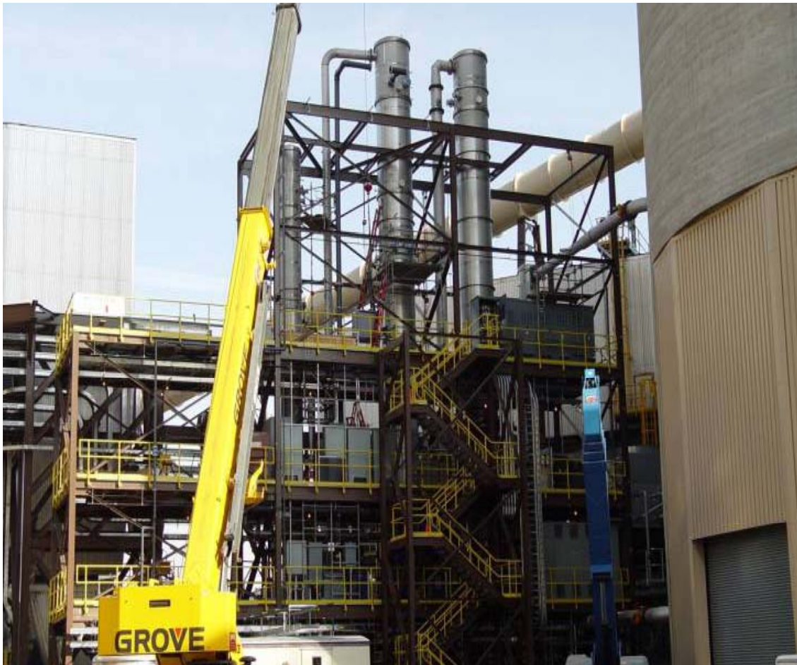
Pleasant Prairie Chilled Ammonia, Post-Combustion Capture Demo Dedicated in February 2008; Late 2007 photo, courtesy of Alstom
