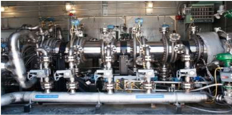
CES 170MW th gas generator
