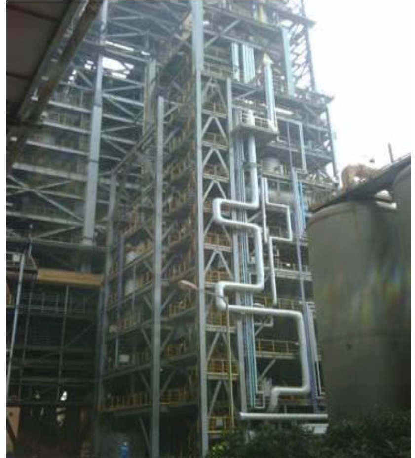
Heat Recovery System
