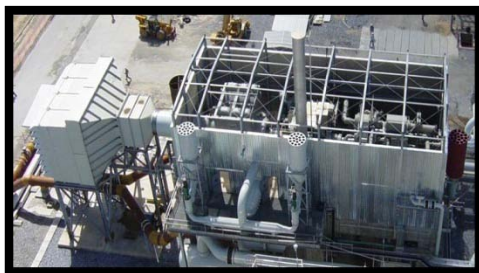
Main and Boost Air Compression
