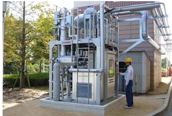
CCU demonstration plant in SAGA, JAPAN (10~20kg/d-CO 2 )
