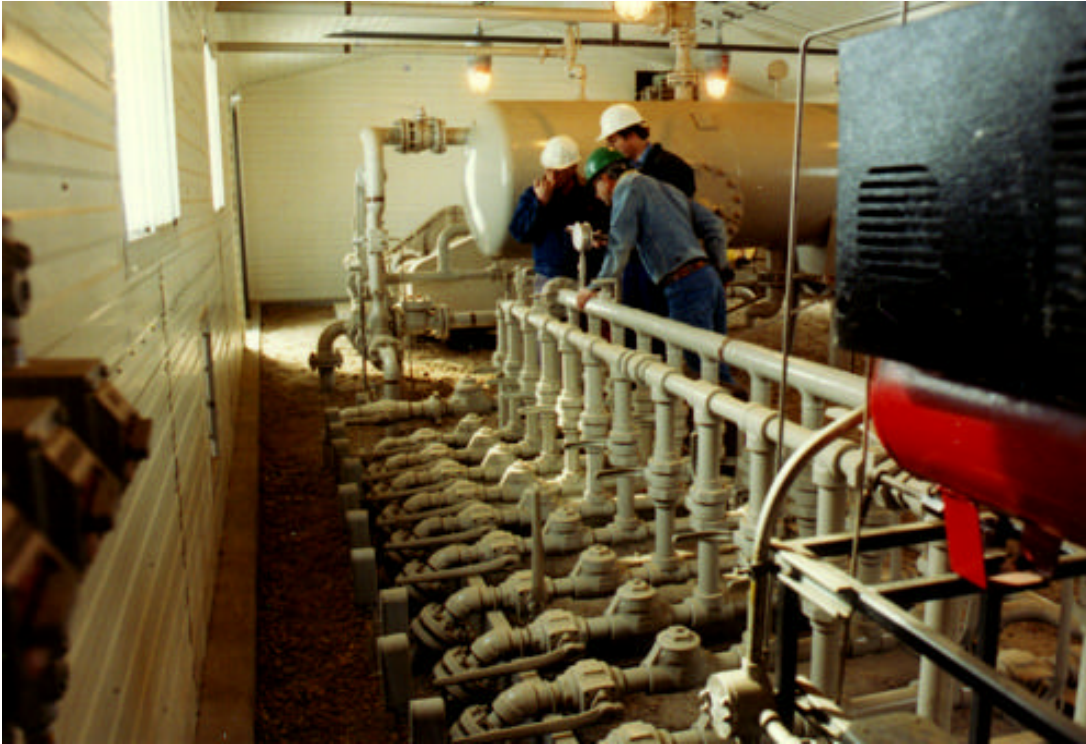
Figure 7 Oil Collection from Producer Wells at Central Automatic Treatment Satellite on Weyburn Field (Courtesy of PanCanadian)
